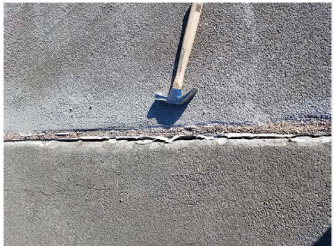
Photo 12 – Failed joint sealant on supported slab.
