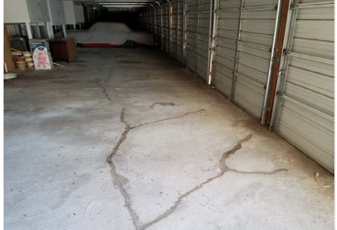
Photo 14 – Cracked and delaminated overlay inside metal building enclosure.
