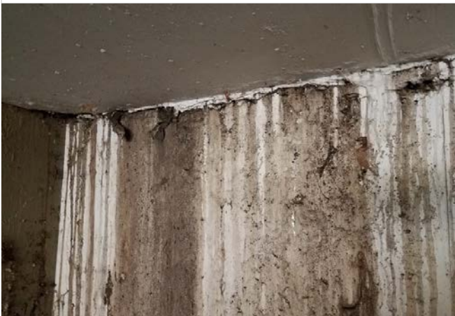
Photo 11 – Stains at perimeter foundation wall indicating leakage through the wall.
