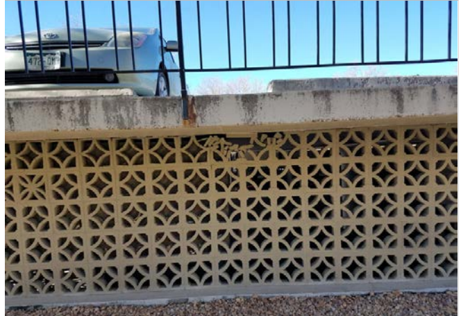
Photo 6 – Damaged CMU light units at top of wall at perimeter foundation wall.
