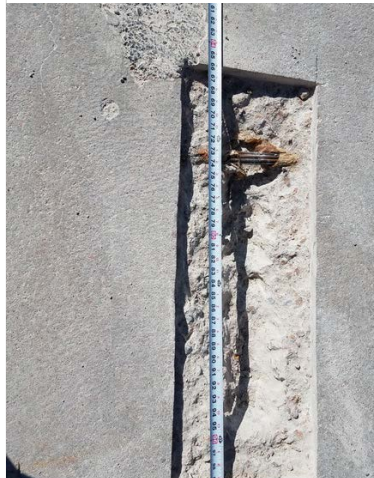
Photo 4 – Corroded PT tendon.
