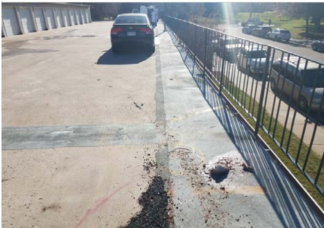
Photo 3 – Traffic coating at the perimeter and asphalt patch material at slab spalling..
