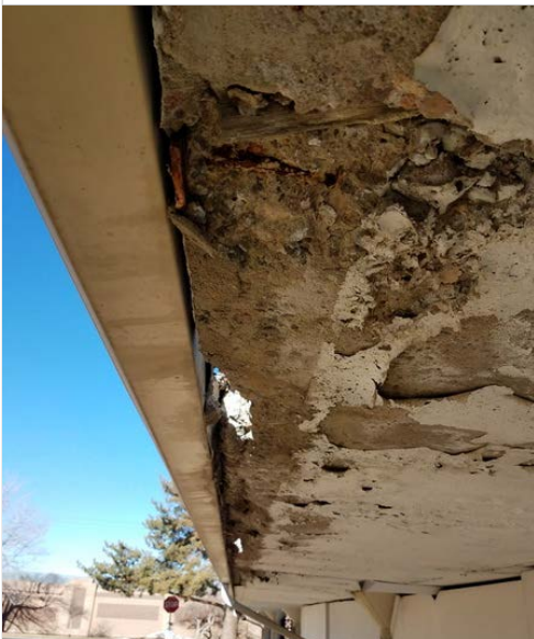
Photo 7 – Severely deteriorated concrete at the west edge of Structure #2.
