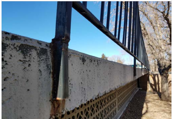
Photo 4 – Perimeter railing with welded post repair and deflection from impact.
