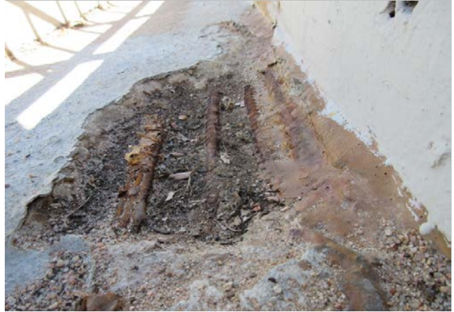
Photo 10 – Spalled concrete at supported slab with corroded rebar and failed PT tendon.
