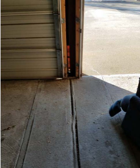
Photo 13 – Failed joint sealant at overlay inside a metal building enclosure.
