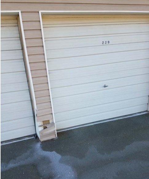
Photo 15 – Damaged siding at meal buildings.
