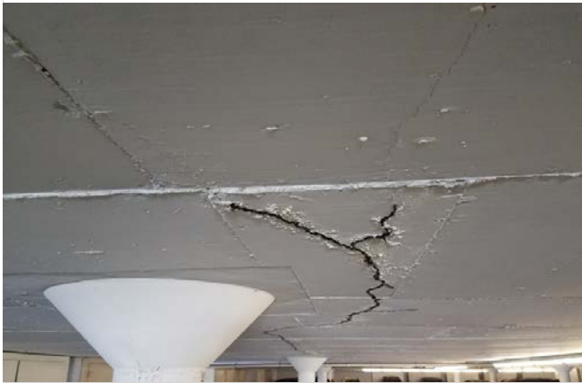
Photo 9 – Crack at parking structure soffit. Note peeled paint and staining indicating moisture migrating through the crack.
