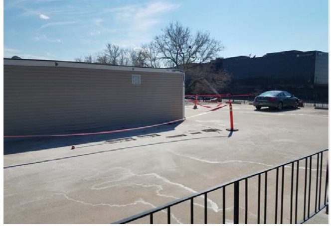
Photo 2 – Exploratory openings of tendons running in the north-south direction.
