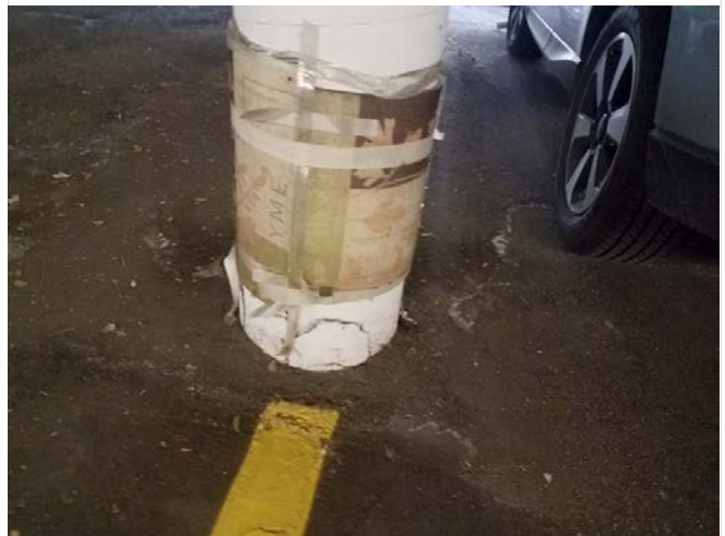
Photo 8 – Typical concrete spall at column.
