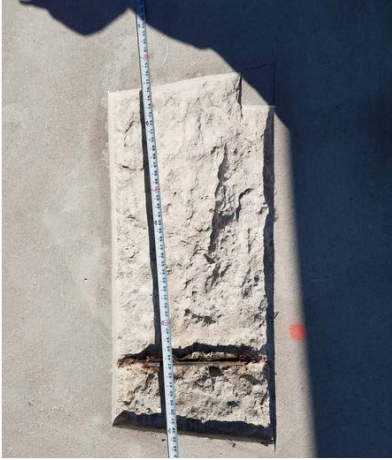
Photo 5 – Severely corroded PT tendon.
