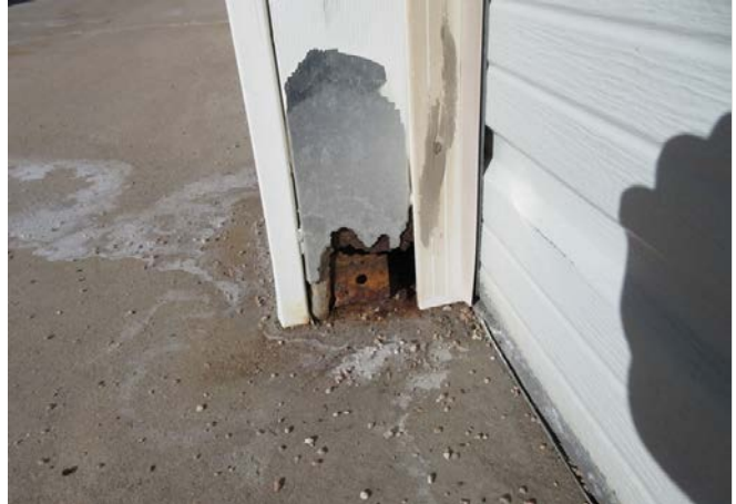
Photo 16 – Damaged façade cladding and corroded structural steel.
