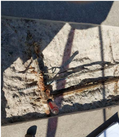
Photo 3 – PT tendon bundles with corrosion present on wires.
