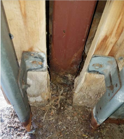
Photo 17 – Corroded structural post and door railings and deteriorating wood framing.
