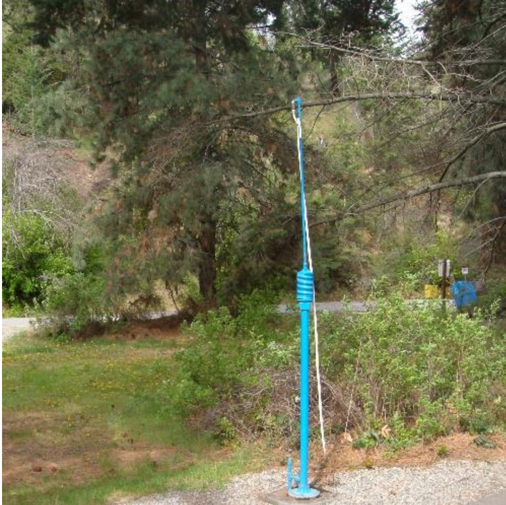
Drinking Water, at this dump station site the rinse water is painted red and the potable water is painted blue
