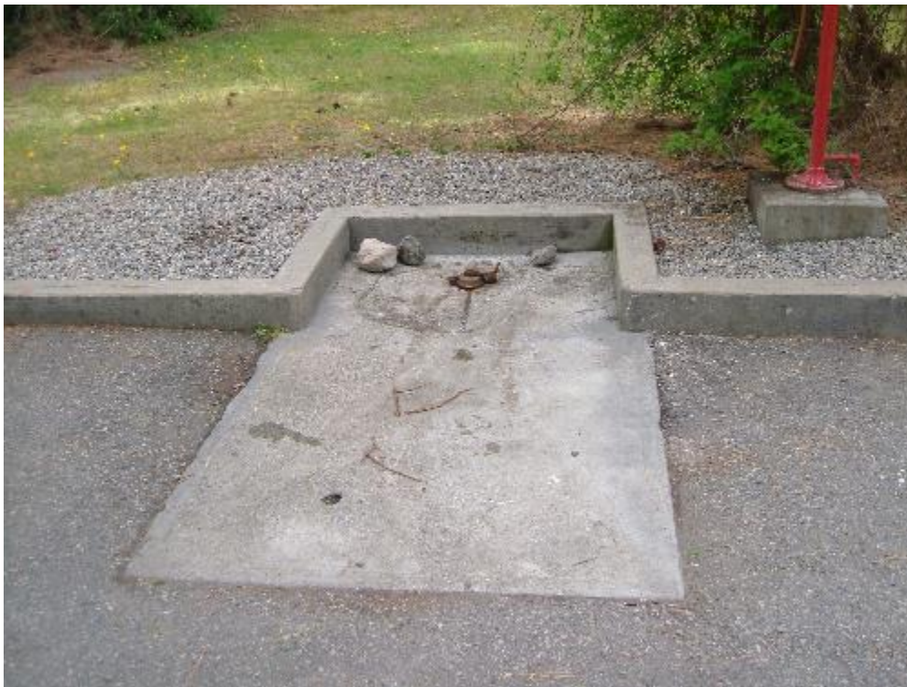
Close up of sani dump drain, notice the slop towards the drain
