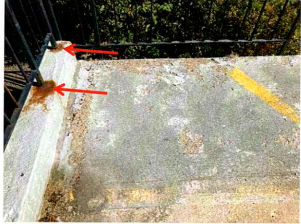
Photo 2: Corrosion at base of posts.
