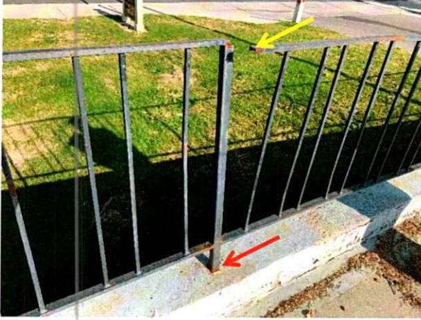
Photo 1: Broken top rail (yellow arrow) and corrosion at base of post (red arrow).
