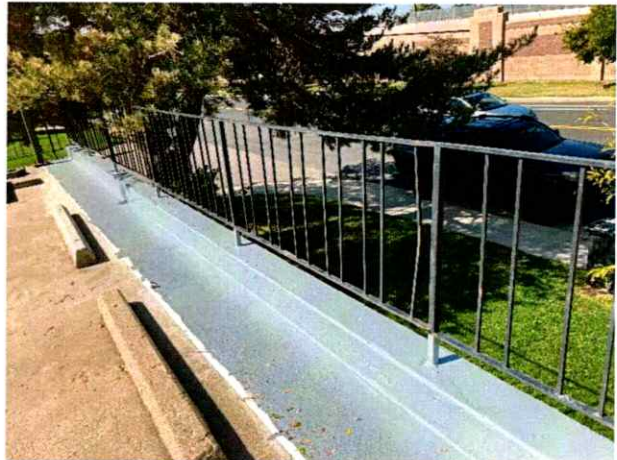
Photo 4: Traffic coating installed over curb and up base of railing post at isolated repair at PS-2.
