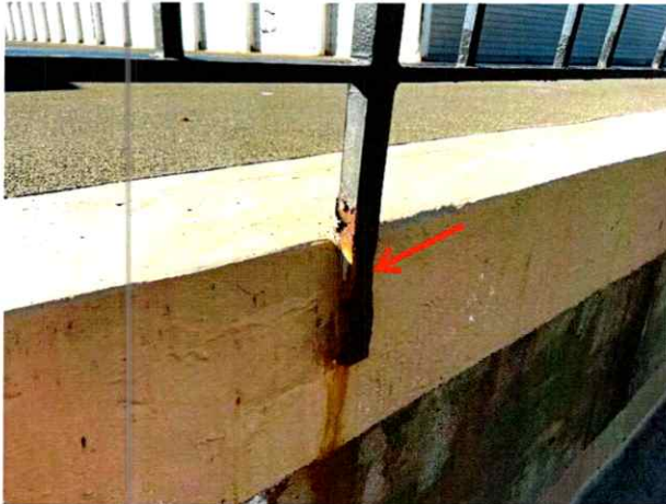
Photo 3: Corrosion and section loss at side mounted post.
