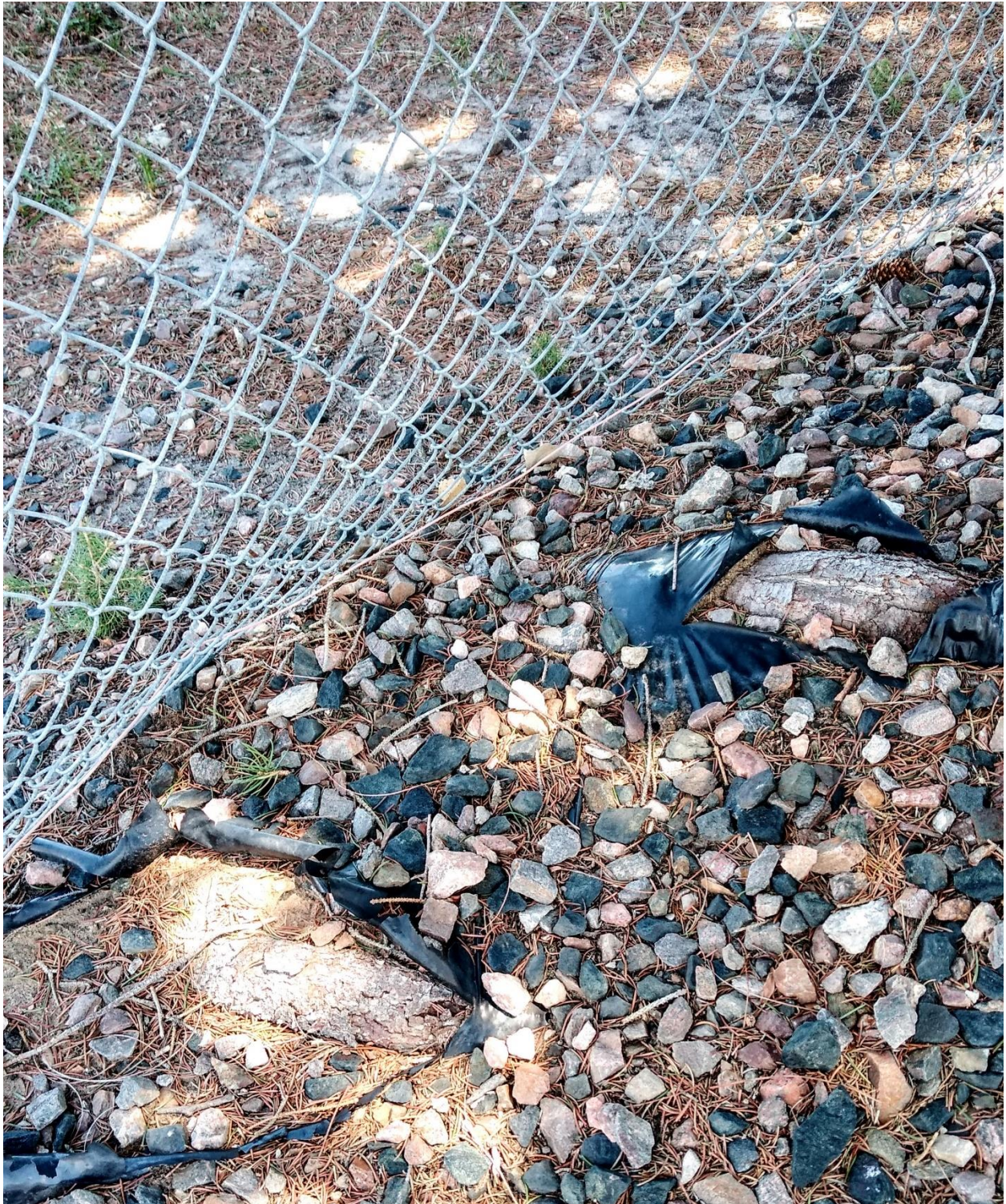
Tree roots buckling fence and that will interfere with the installation of the new fence.
