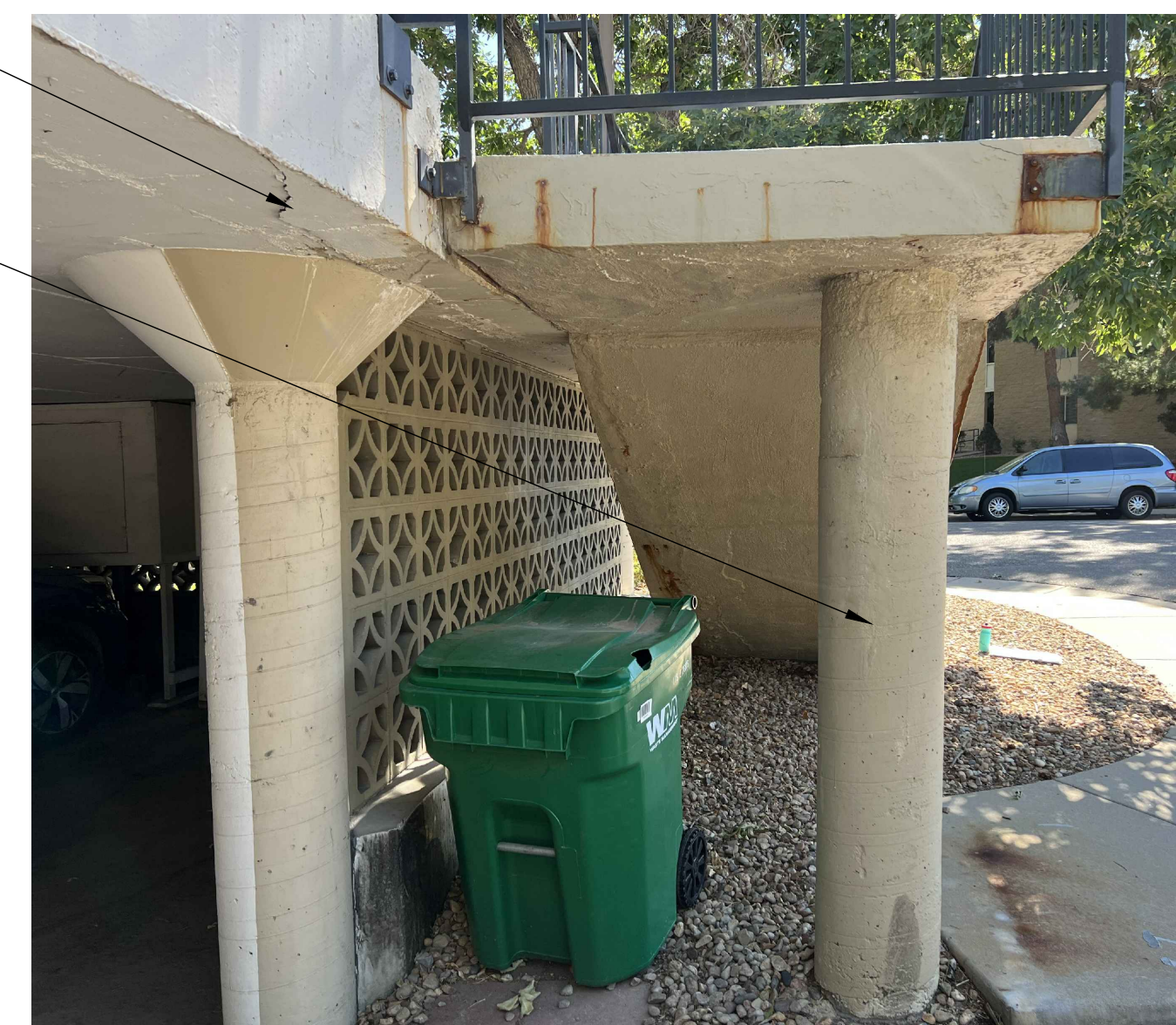
DETERIORATED SLAB EDGE
